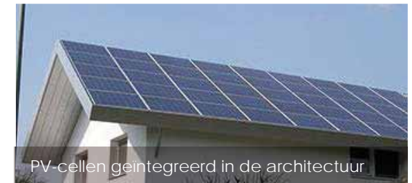
PV-cellen in nette, regelmatige vlakken
